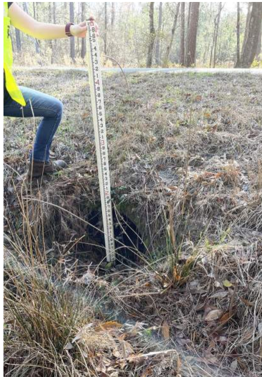
Figure 45: Crossing #2 along John Carter Road. The level rod is rested on the approximated 12" of sediment accumulation at the invert of the 24" RCP. The view is facing downstream.
